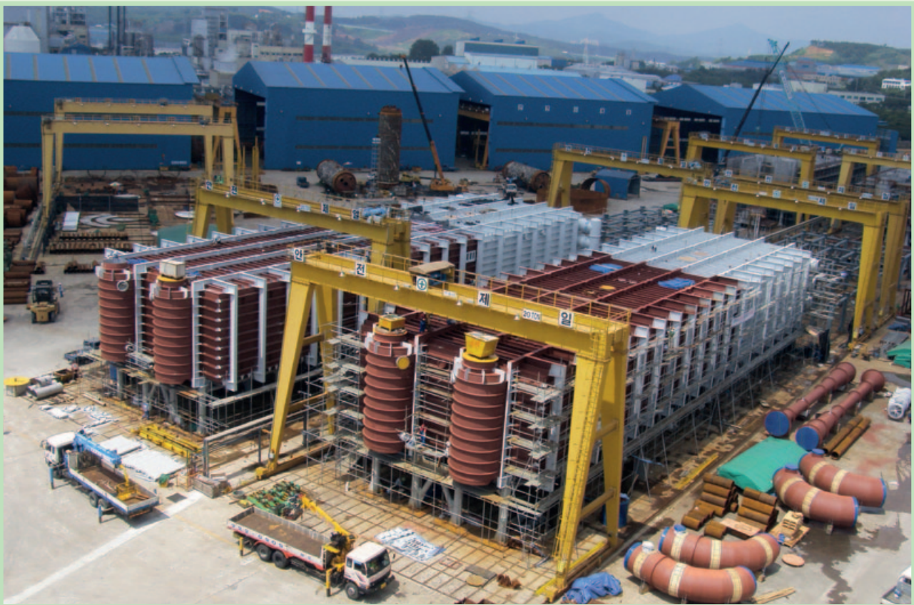
MED type evaporator of Marafiq IWPP in Saudi Arabia Photo: Sungjin Geotech. Co.]
