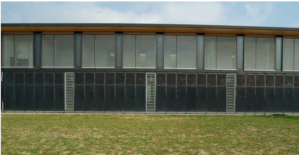
Fig. 25: Thermal solar façade made with absorber for heat exchange from solar radiation to liquid (Energie Solaire, I. Frei).
