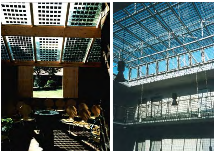
Fig. 17: Winter garden (left) and atrium glazing (right) in combination with semi-transparent photovoltaic roof elements (solarnova).
