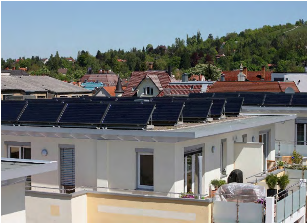
Fig. 28: Support structure for thermal collectors (Buderus)
