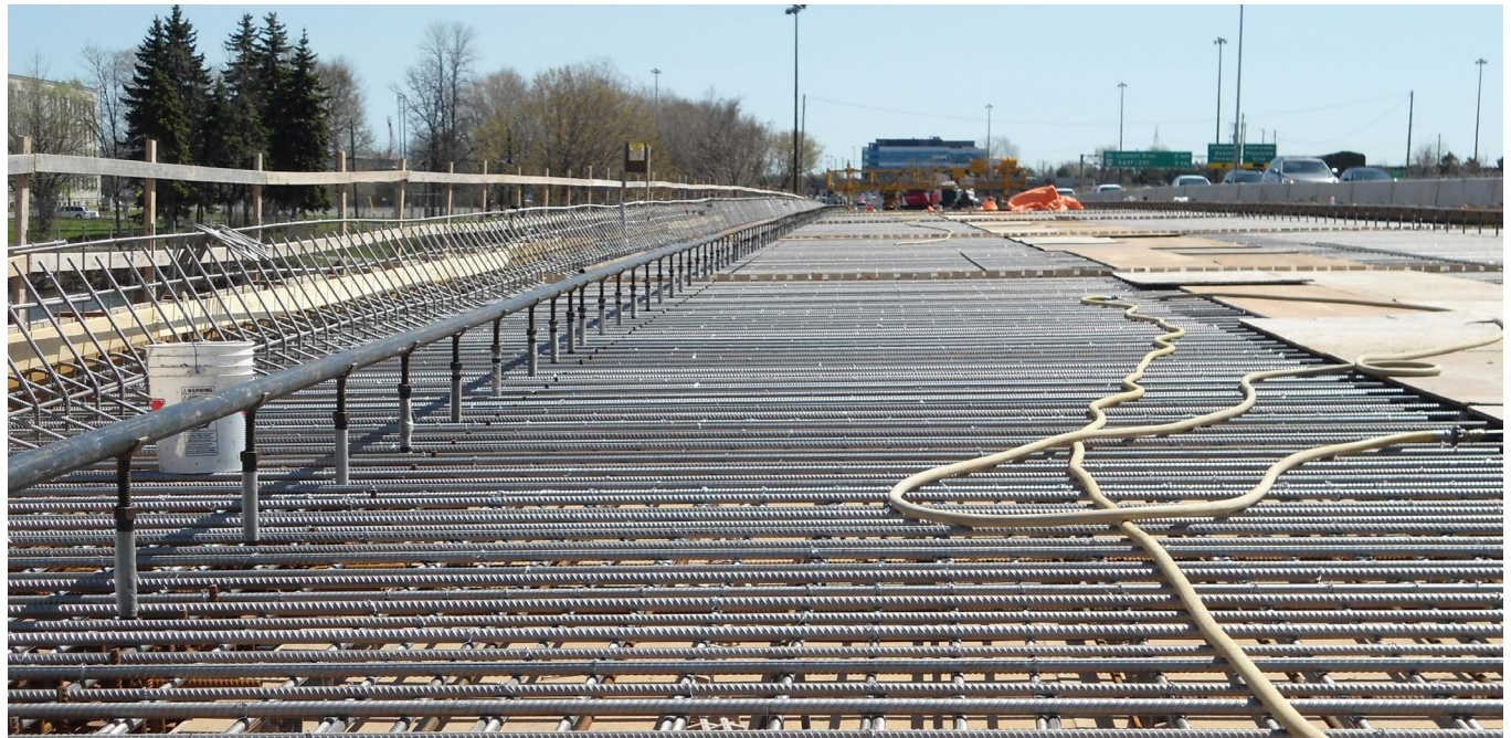
Where de-icing salt is used in winter, stainless steel reinforcement is an advantage. Photo: Frank Smith
