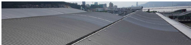
Stainless steel grade 316 is used in the building envelope of the extended Macau Taipa harbour terminal.
