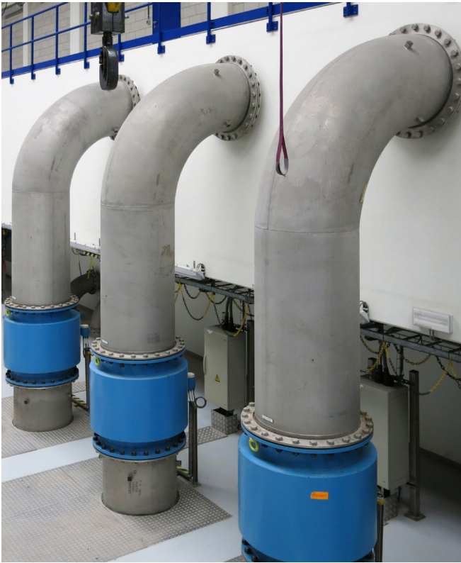
In waste water plants, stainless steel defies the combined effect of corrosion attacks and abrasion.
