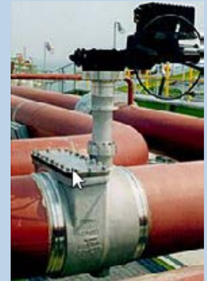
Valve at the LNG terminal in Bilbao, Spain
