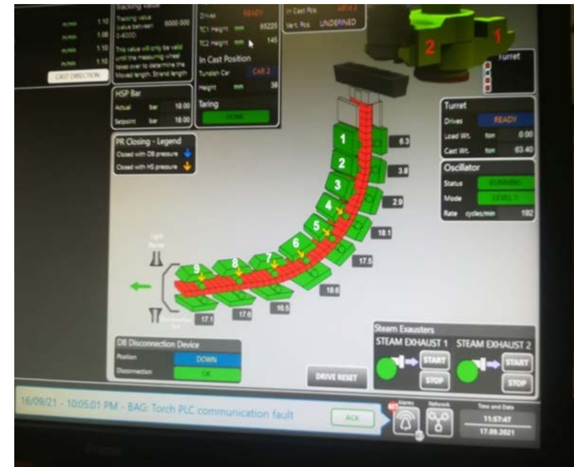
| CCM Segment working area
