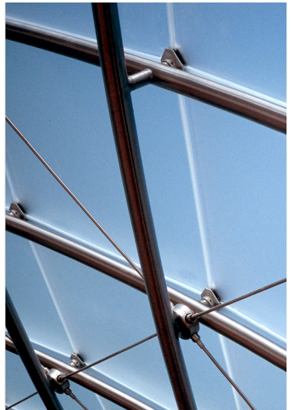
Figure 2: View of the stainless steel members and node point in the band shell (Photo: James Carpenter Design Associates and Shane McCormick)
