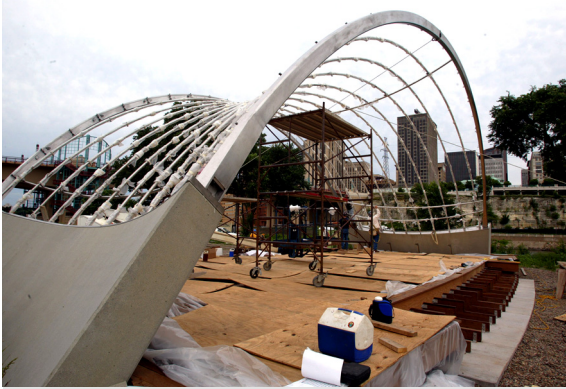
Figure 6: Installation of the curved edge beams and lattice members (Photo: The Schubert Club)
