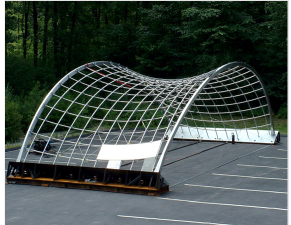
Figure 3: The Band Shell was first put assembled in the fabricators car park to ensure a good fit-up (Photo: Tim Eliassen)
