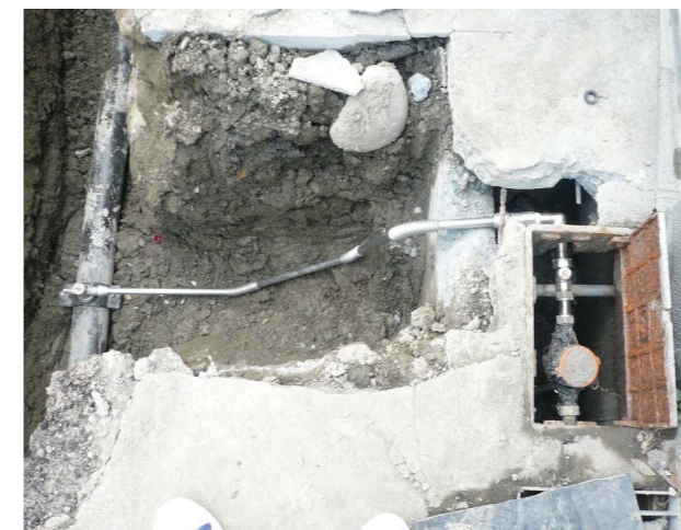
SPCT is simply bent at the corrugations to fit the installation, avoiding buried fittings and joints.
