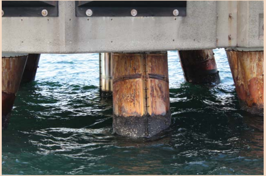
Steel pipes which have not been protected with super austenitic stainless steel jackets
