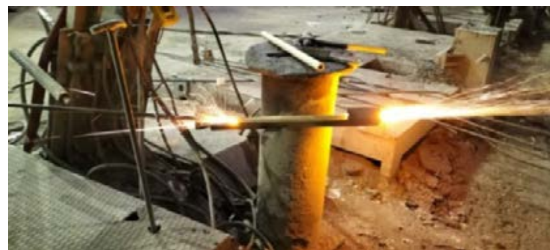
Fig. 5. New method developed for the ignition of the oxygen lances. This procedure avoid the risk of burns and contact with hot substances for the operators
