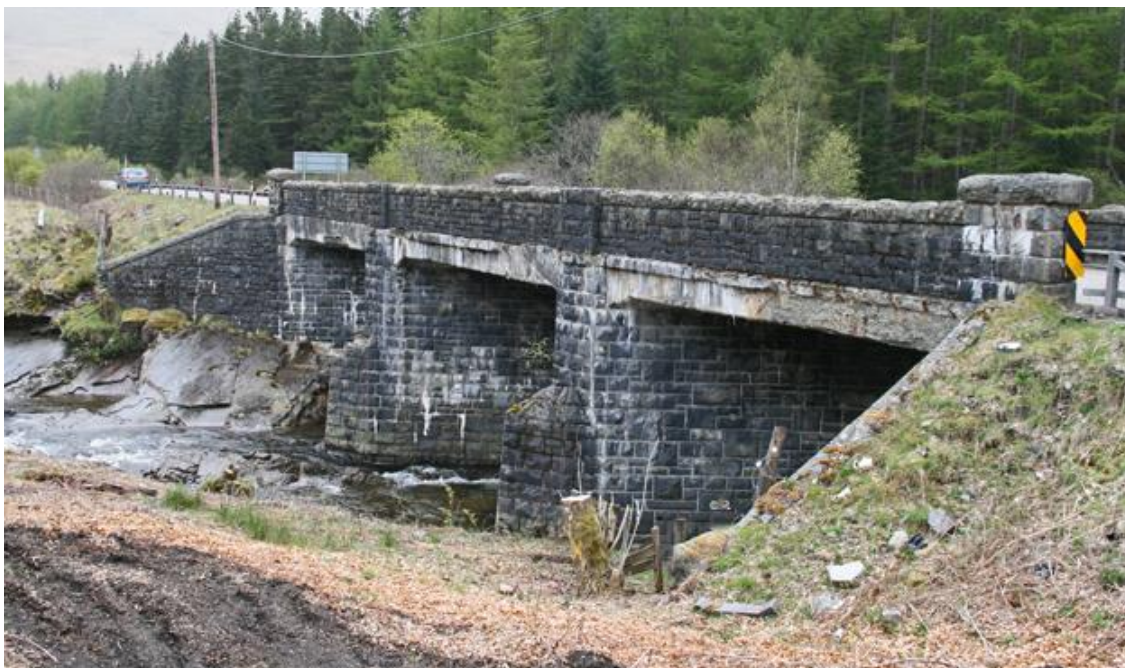
Original Allt Chonoglais Bridge prior to demolition and showing signs of rebar corrosion
