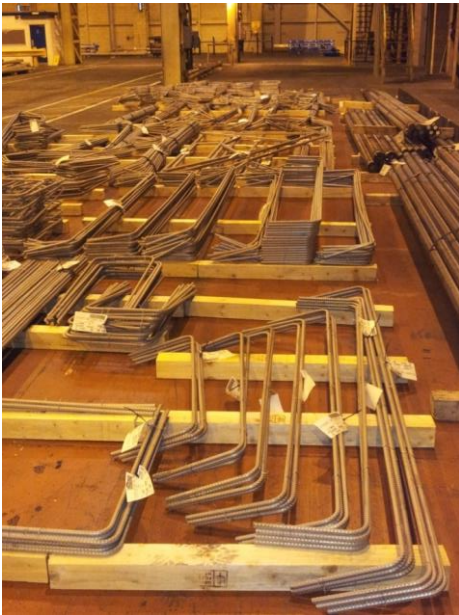
Stainless steel reinforcement having been fully cut and bent at Outokumpu's Sheffield Stainless Bar facility
