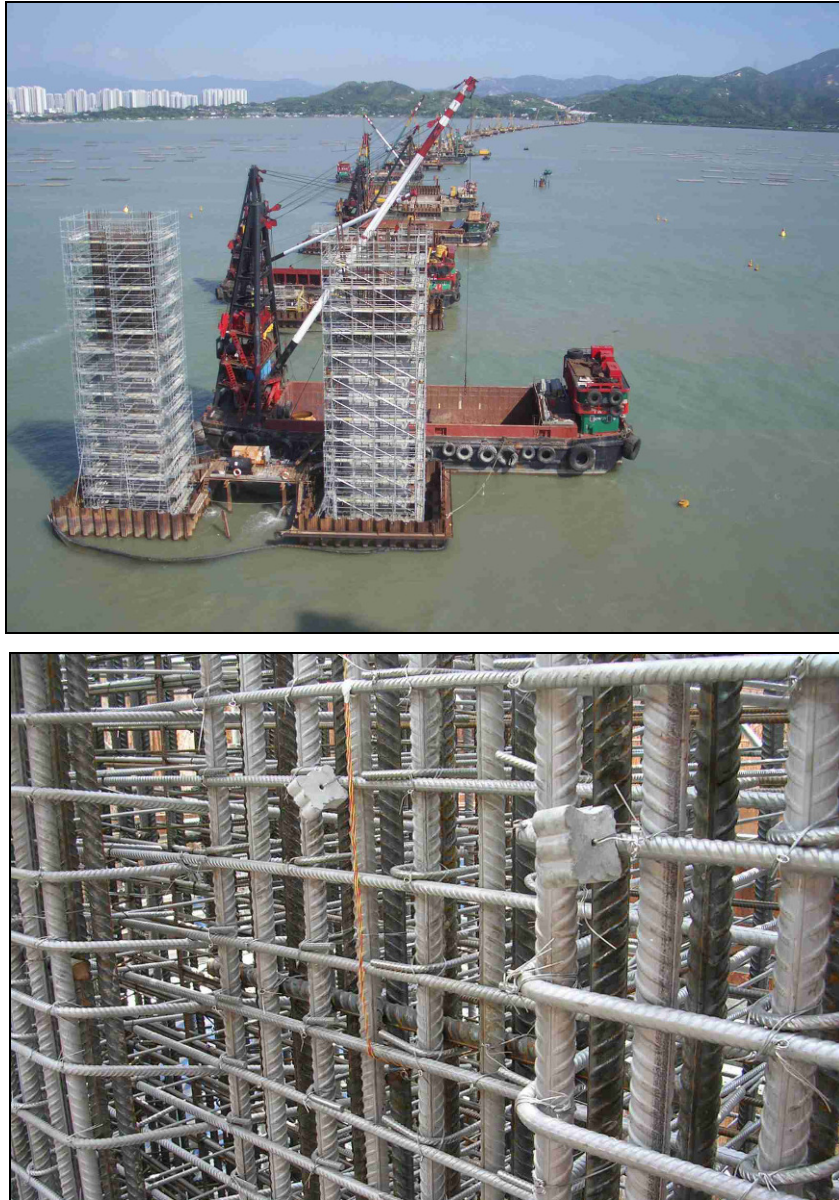
Figure 7.2 Stainless steel reinforcement on the Shenzhen Western Corridor
