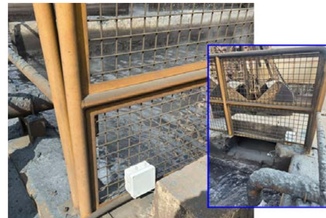
Installed IOT dispositive.
